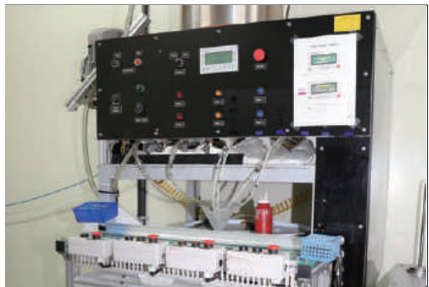
Oil filling station for P6
